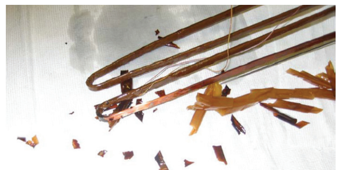
Aged and brittle conductor insulation (photo by DuPont)
